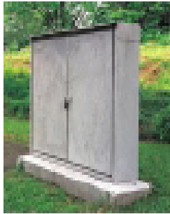
An over-ground box is one of several indications of the presence of underground electricity cables.
