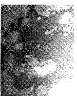
劣化部位の噴霧の様子 Side view of deteriorated parts
