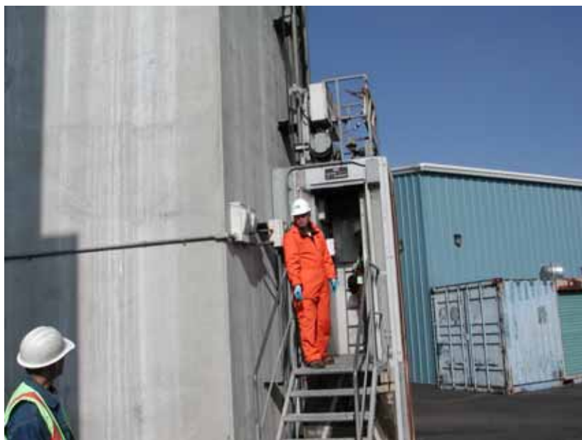
橋梁於墩柱附設檢查之升降電梯
