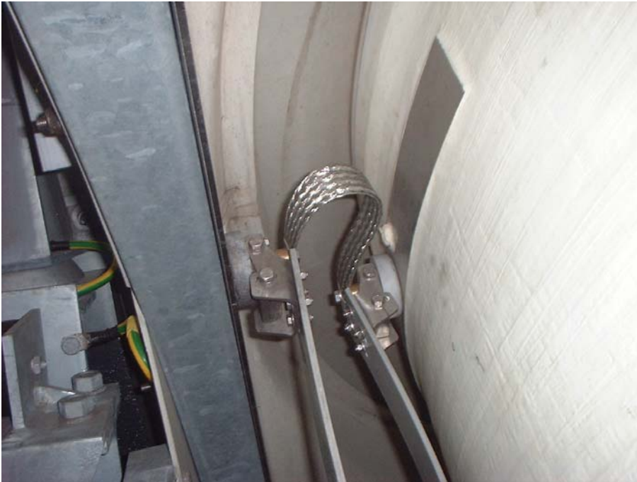
Figure 4 LCTU between blades and nacelle chassis
