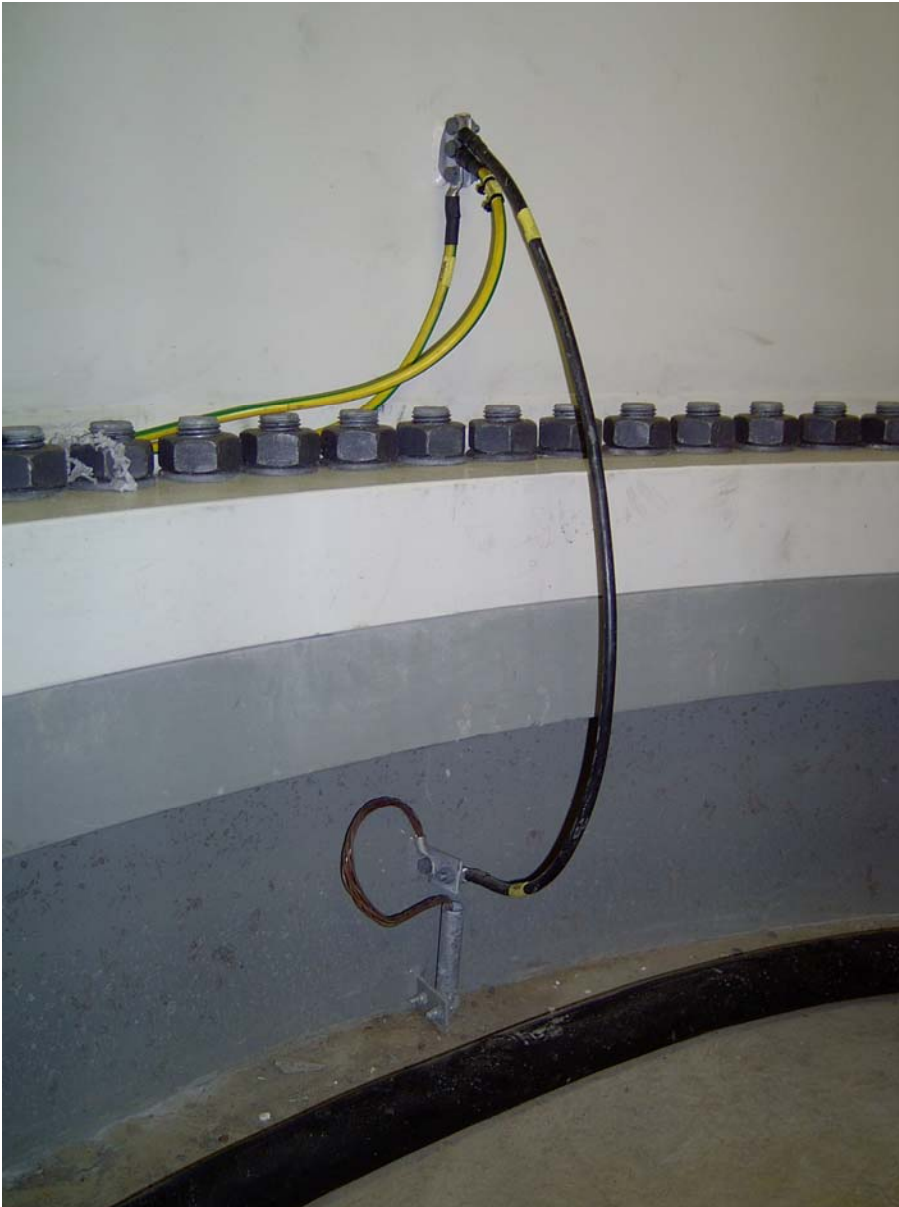
Figure 7: Connection between the earth distribution cables, tower and external earthing system.
