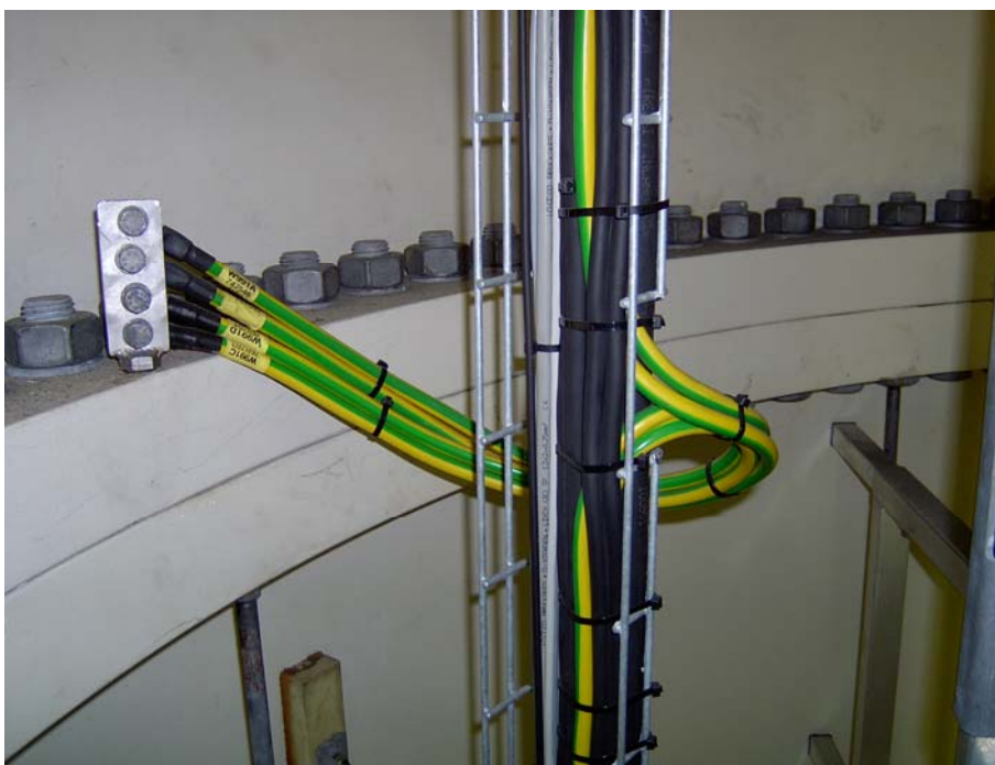
Figure 6: Bonding of down conductor from the nacelle to the base of the top tower section.
