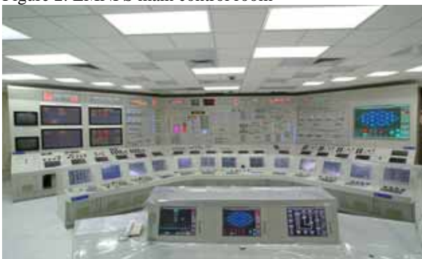
Figure 2: LMNPS main control room
