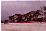
Figure 2: Collapsed condominiums along Orange Beach, AL following the landfall of Hurricane Ivan.
