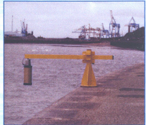
The radar tide gauge at Liverpool, similar to that planned for Gibraltar.
