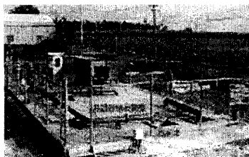
Fig.10 Aquifer Storage and Recovery (ASR) Demonstration Site, Pingtung County
